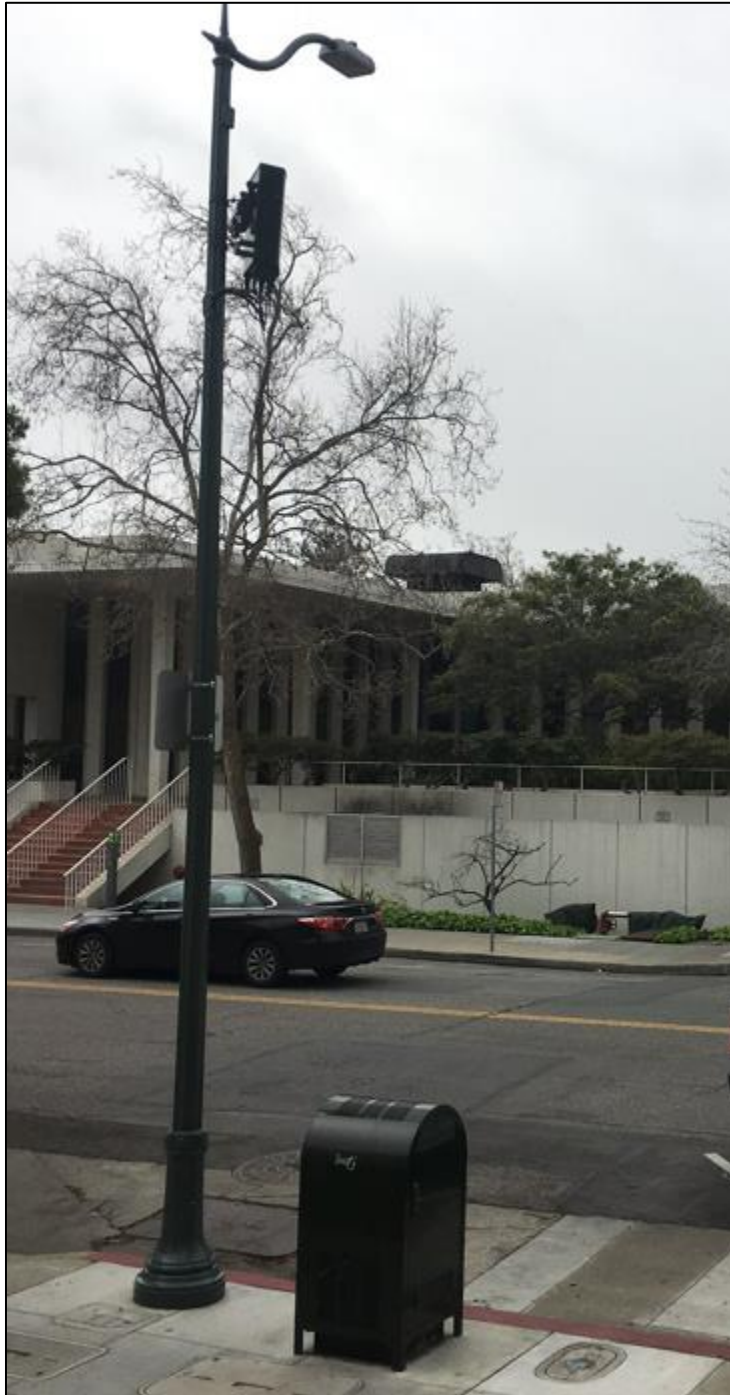
Figure 9: Ground-mounted accessory equipment concealed as a mailbox.
